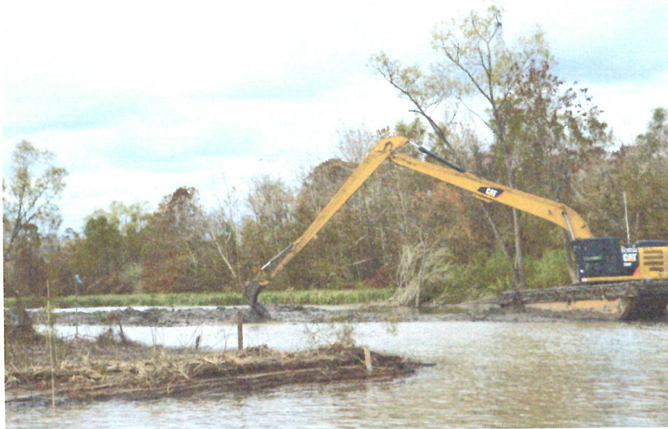
Figure B: This photo was taken by Dean Wilson during the monitoring trip in the Basin on December 7, 2018. This photo was taken in the same location as Figure A. This photo depicts active construction in the area and again, a lack of erosion or sediment control measures in place.
