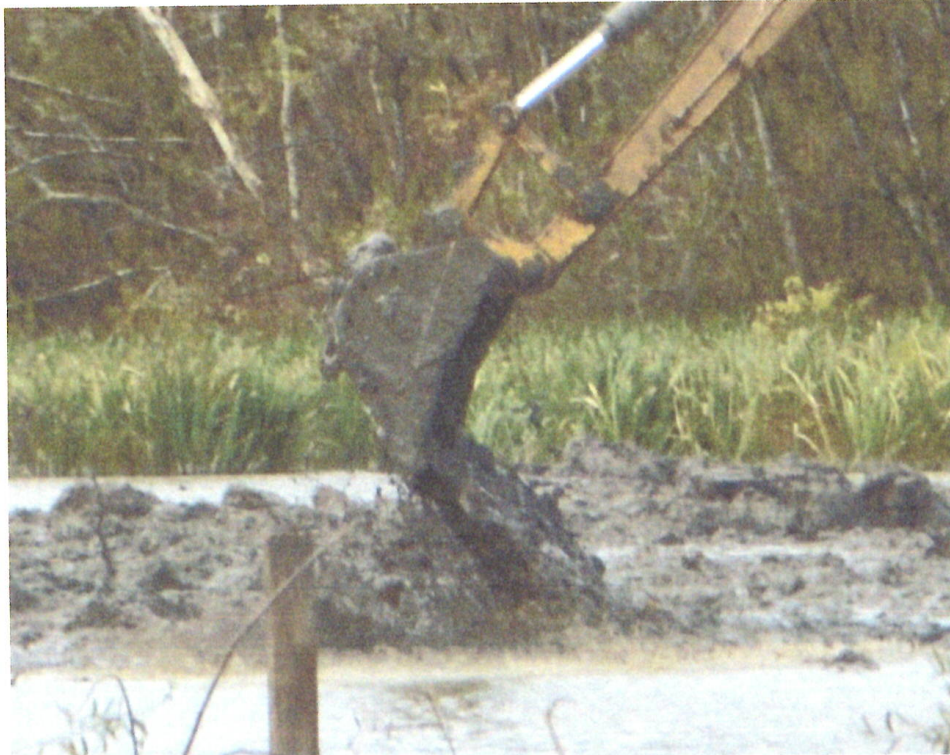
Figure C: This photo was taken by Dean Wilson during the monitoring trip in the Basin on December 7, 2018. This photo was taken in the same location as Figures A and B above. This photo more clearly depicts the discharge of mud from construction.
